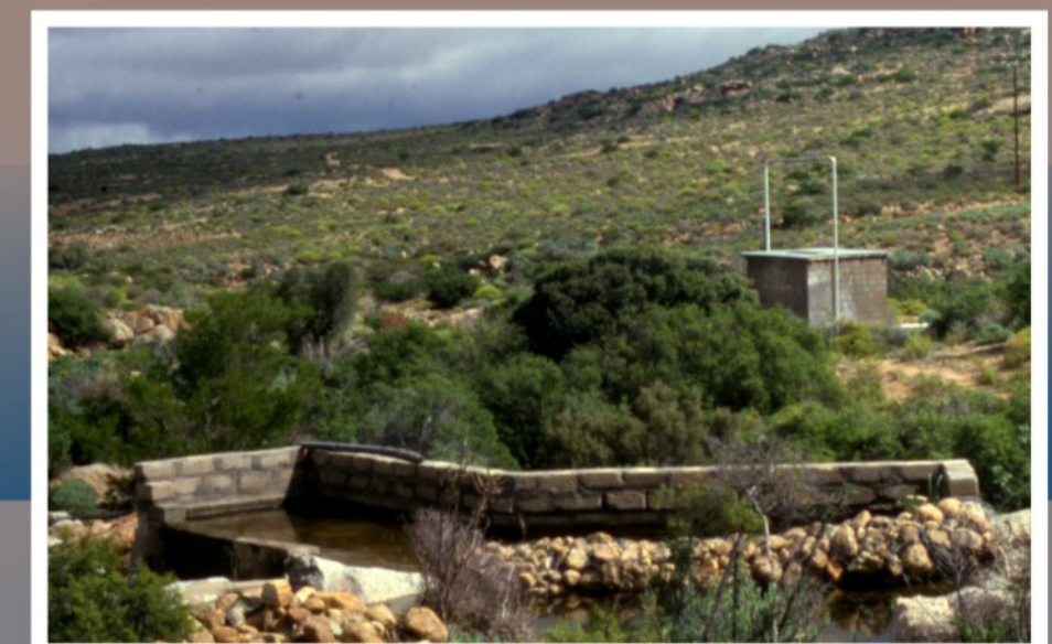
Sand filter and injection/ abstraction borehole, Namaqualand, RSA
