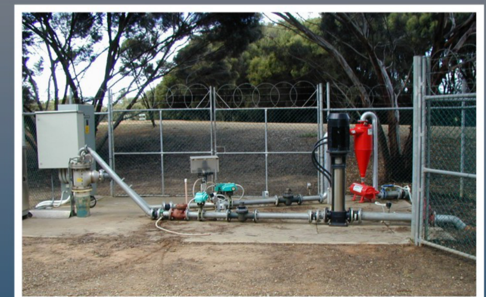
Injection/ abstraction borehole, Adelaide, Australia
